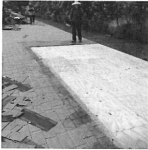
Open Patio Covered by Mutual with city permit prior to roofing
