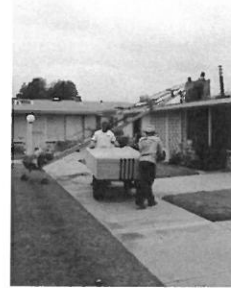
Buildings without drive up access wheel on cart to conveyor
